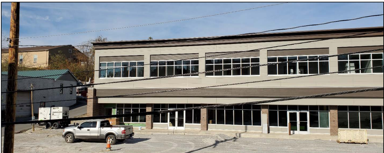
An under construction commercial building approved through a Variance and Land Use Permit
