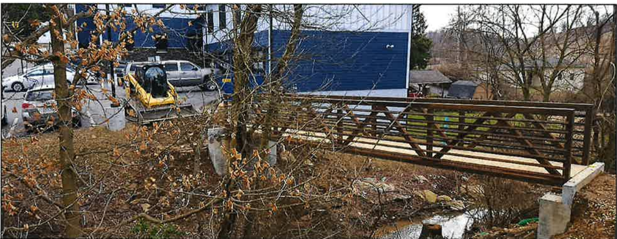
Under construction accessory walkway bridge approved through a Land Use Permit on 12-18-2017
